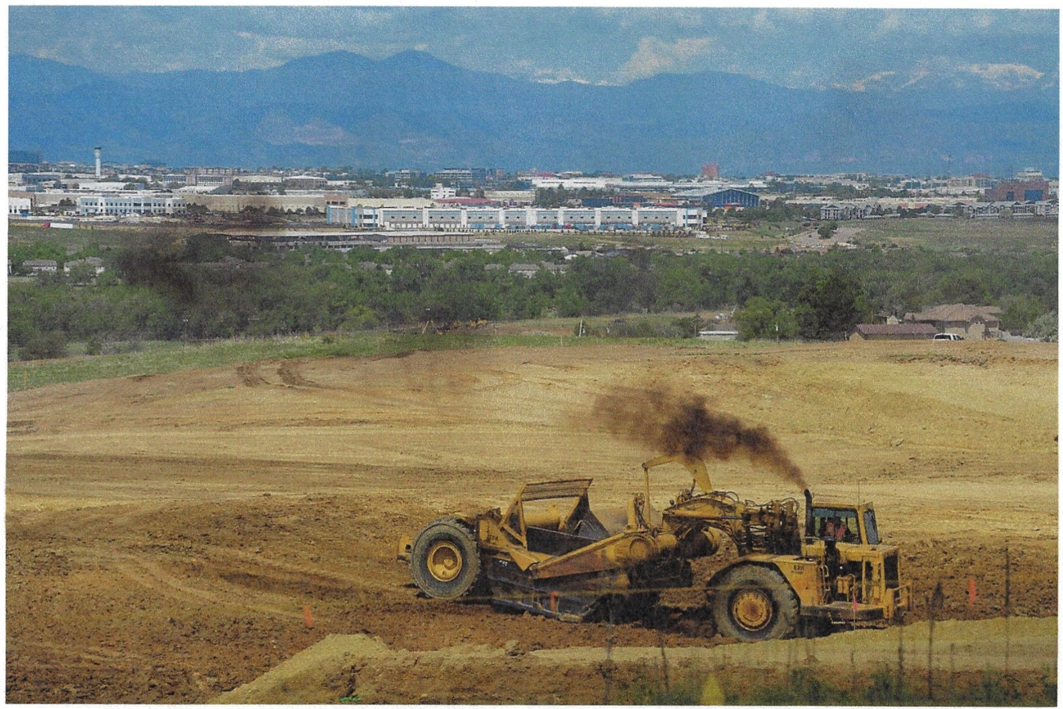
Workers clear land Thursday in preparation for homes and a golf course to be built at the new Prairie Point master-planned development built by Oakwood Homes in Aurora. Oakwood Homes expects nearly 1,600 homes to be built by 2028. PHOTOS BY HARMON DOBSON — THE DENVER POST
