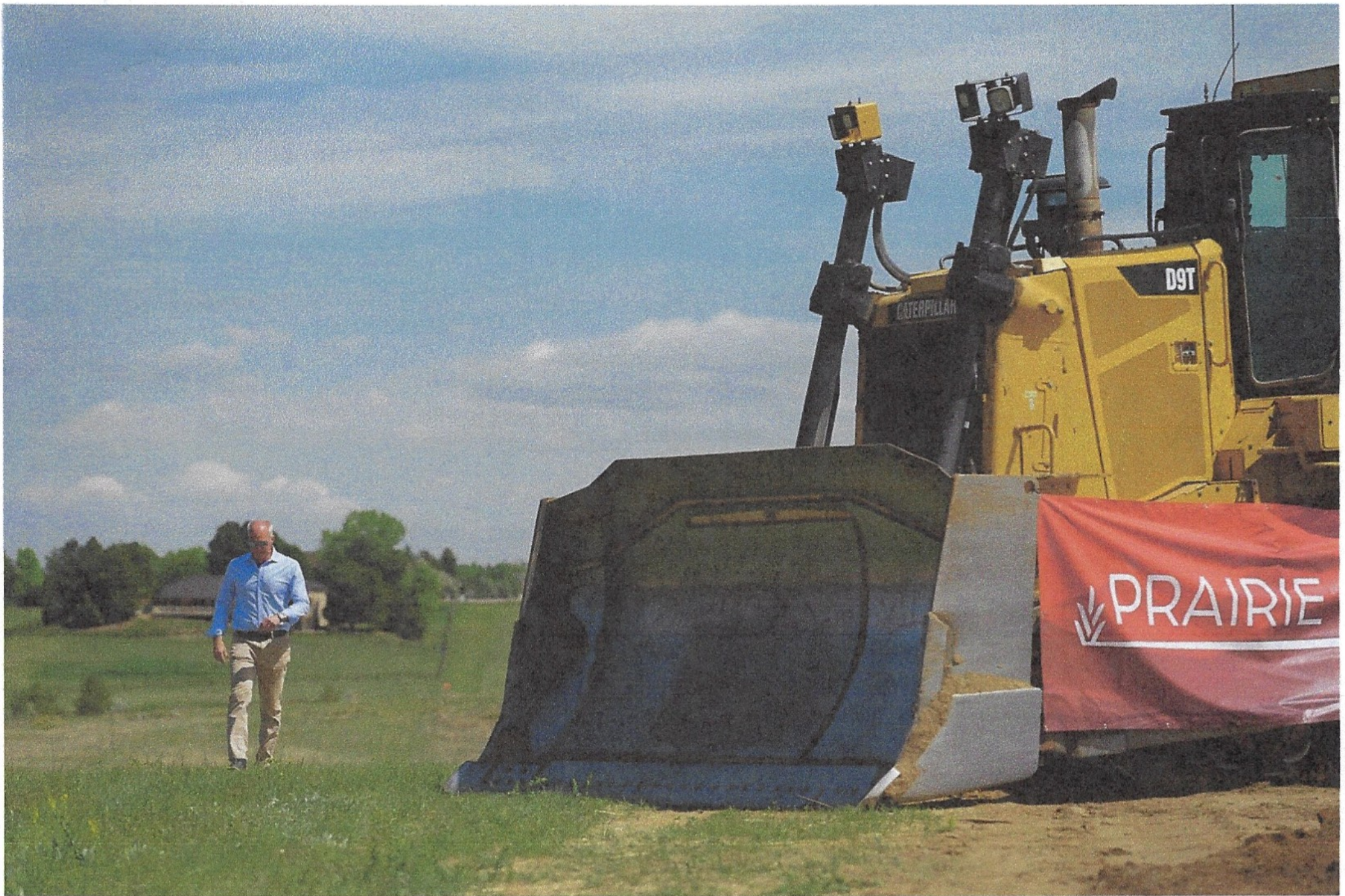
Todd Bloom of Oakwood Homes walks next to a heavy-duty dozer at the Prairie Point site.
